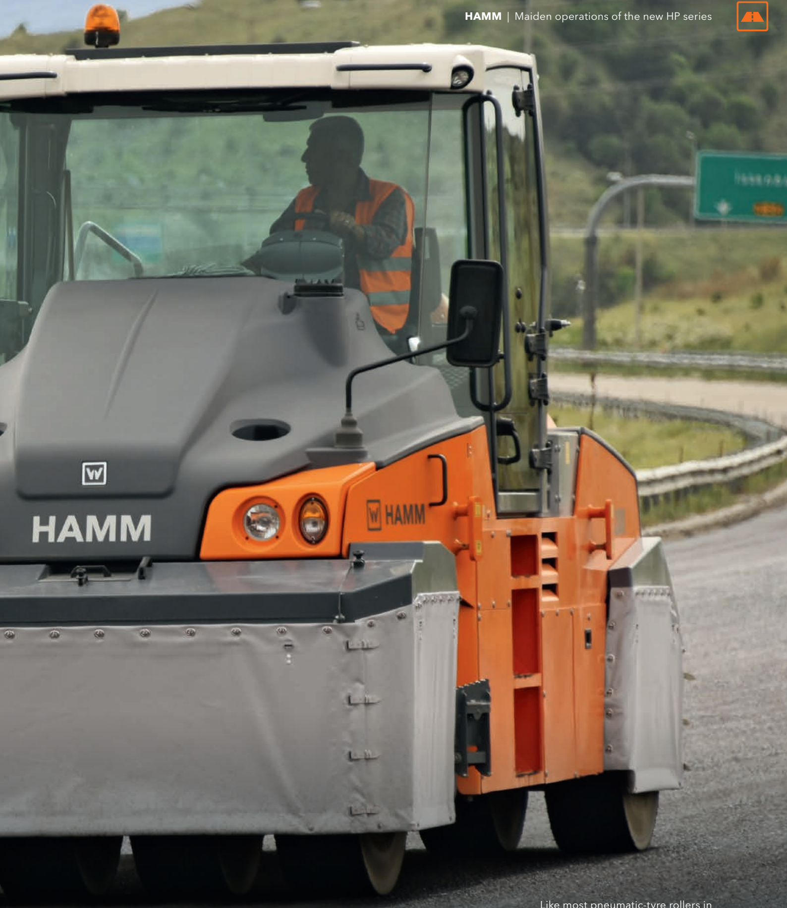
Like most pneumatic-tyre rollers in Turkey, the HP 280 used near Ankara was fitted with thermal aprons.
